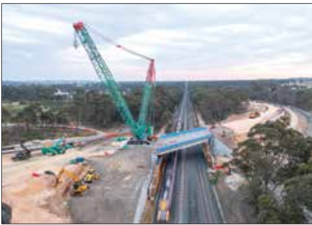
PROGRESS: The Inland Rail project has reached a new milestone with the installation of bridge beams over the rail corridor at Seymour-Avenel Road.
